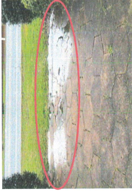
Front Sidewalk – broken tile, standing water due to settlement of sidewalk and age of material.
