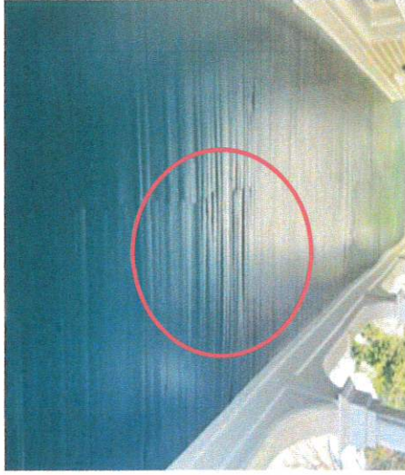
Front Porch Ceiling – showing the results of water damage.
