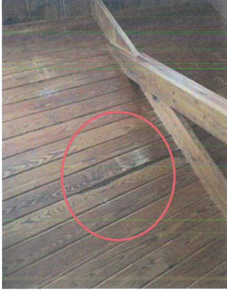
Sunroom – showing the result of water damage to interior ceiling due to the roof leaking
