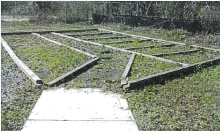
Not Acceptable No fence; overgrown with weeds.
